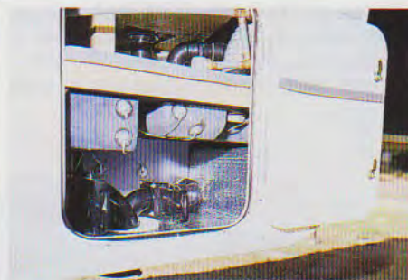
The enclosed heated holding tank system.
